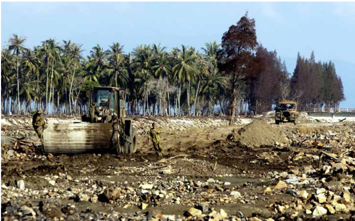
Sappers from the Australian Army 1st Combat Engineer Regiment lay beach matting across soft ground to open the road from the landing point into Banda Aceh, Indonesia, for tsunami relief and reconstruction operations.
