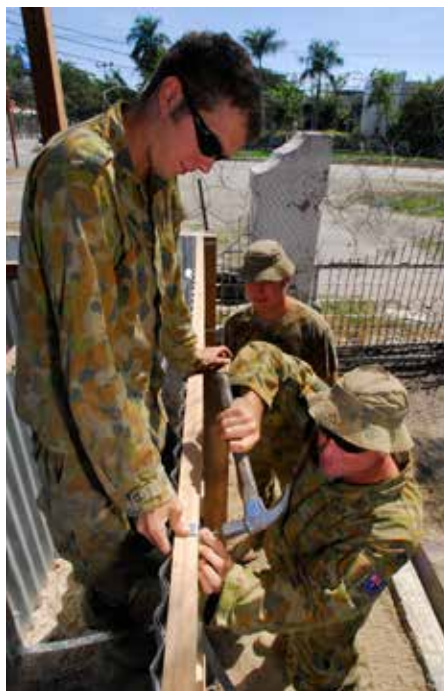
Sappers from the 3rd Combat Engineer Regiment build a strong point at the front of Camp Phoenix, Dili.
