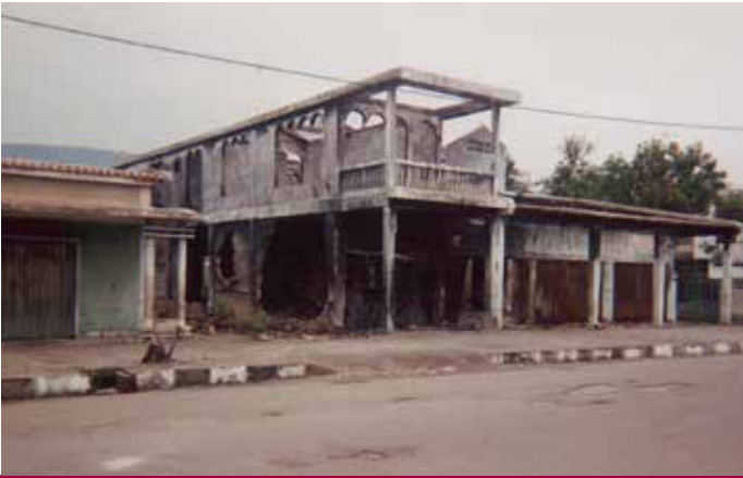
A shop front with accommodation that was destroyed by fires set by the 'Militia' in late 1999 during the 'consultation' period for ET's attempts to gain independence from West Timor and Indonesia
