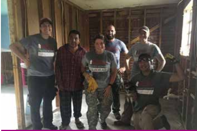
Ms Fenton and her team spent eight days repairing houses in Houston. (All pictures supplied: Deborah Fenton)
