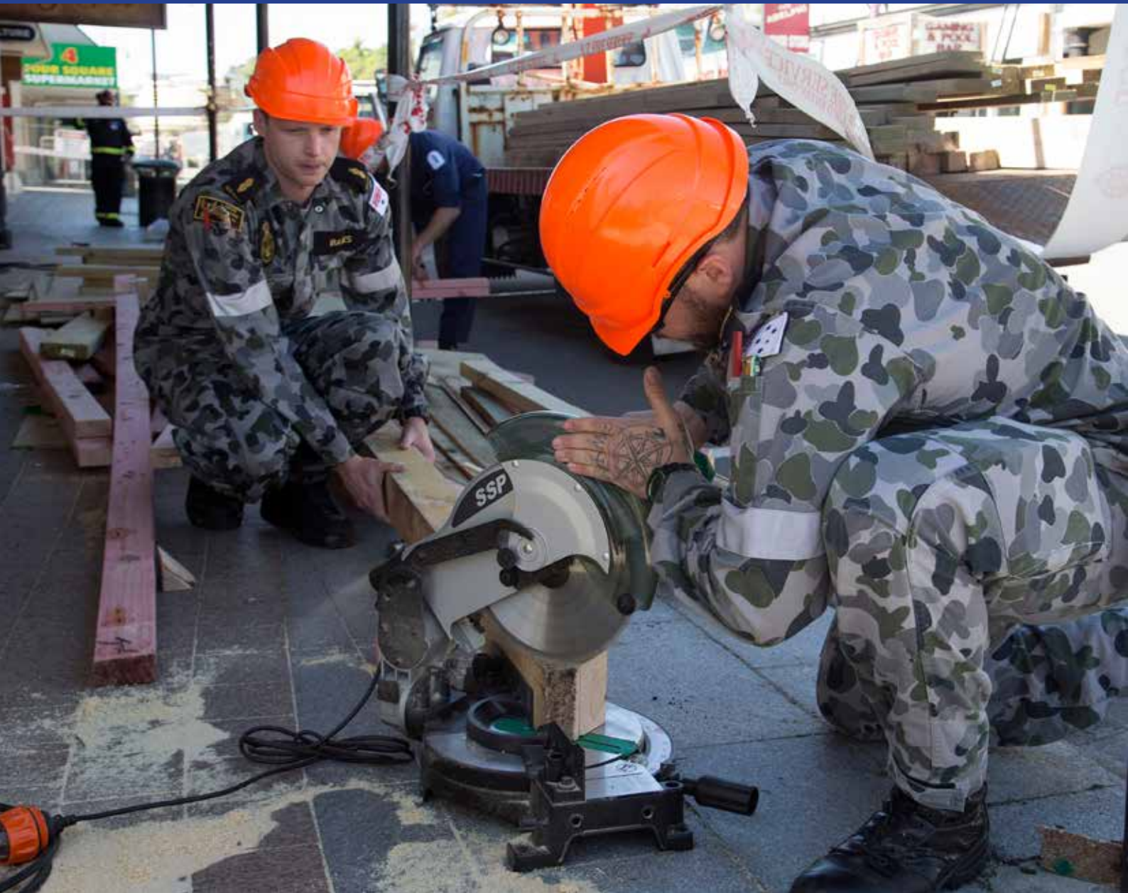
Below: Able Seaman Electronics Warfare Nicholas Bates (left) and Leading Seaman Electronics Technician Vincent Carroll cut shoring to reinforce a wall in the township of Kaikoura.
