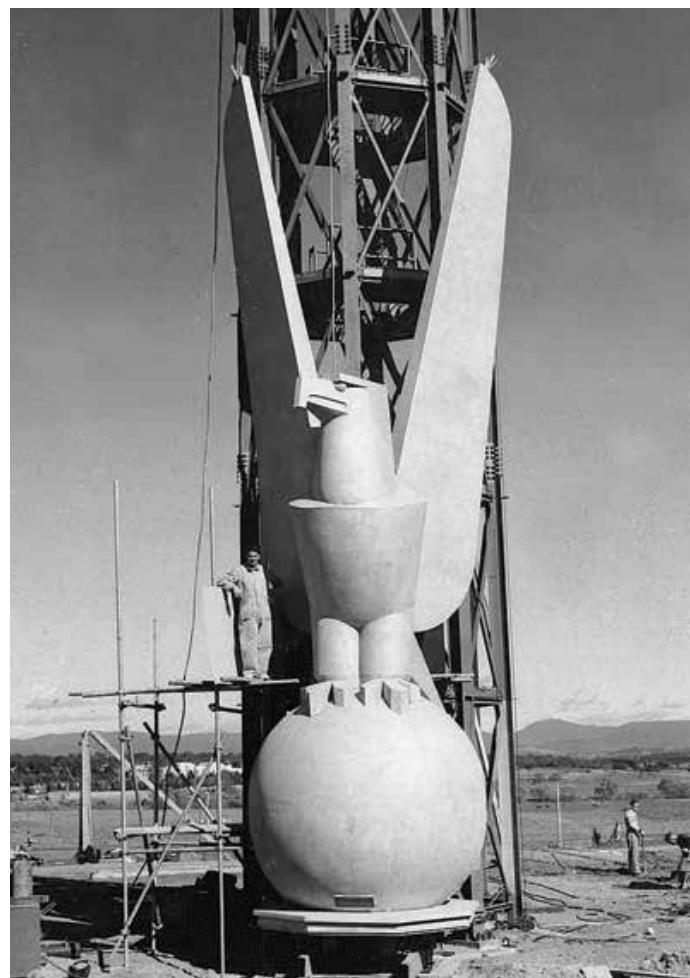
The Eagle, designed by sculptor Paul Beadle, is ready to be hoisted to the top of the memorial.
